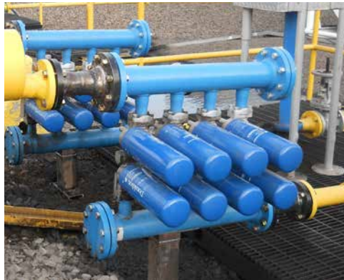
Single-pass Bulk Fuel Filtration System
