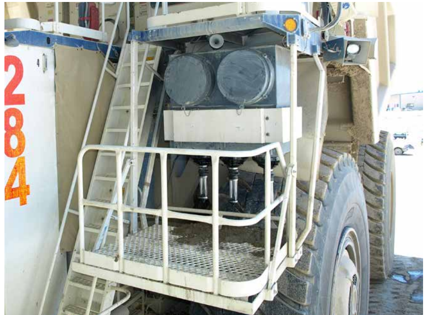
Dust Dumpa kits installed on a Donaldson SSG29 with rain shields. Notice the piles of dust gathered on the platform during vehicle operation.
